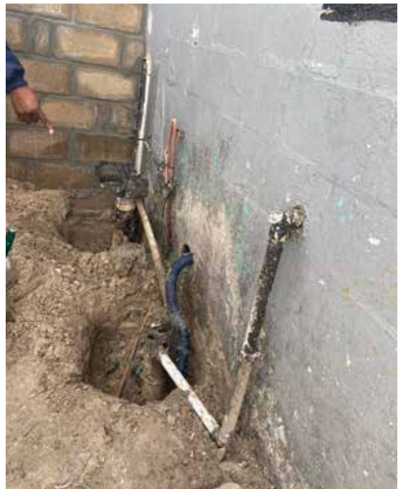
Pictured above: Corroded and worn sanitation pipes before installation.
